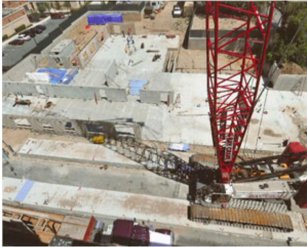
Original design plans were modified to create a precast concrete structure with hollow-core plank floors, interior bearing walls and precast concrete staircases.
