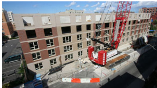
The complex is being built on East 156th Street between Melrose and Elton avenues in the South Bronx. The one-, two- and three-bedroom units are for families with incomes below 60% of New York City's adjusted median income.
